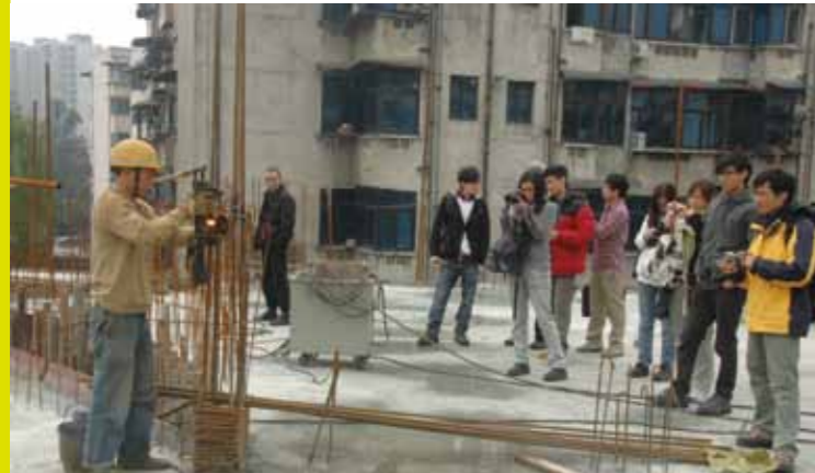
Students from the Faculty of Engineering frequently visited the site to gain first-hand experience of construction and supervision in the Project Mingde
